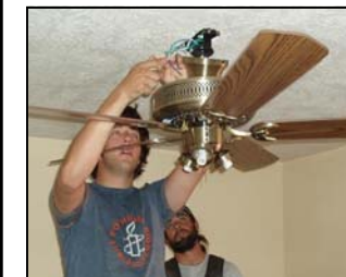
Gianni B. installs a ceiling fan with the help of Kenny a licensed electrician.
